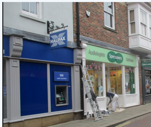
Regular maintenance regime
