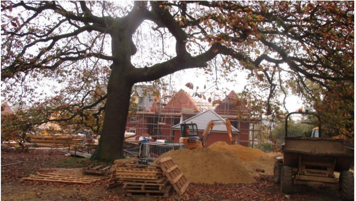
Figure 14. Bad practice: construction activities within the CEZ | DCC
