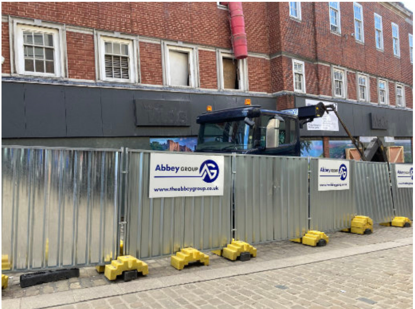
The disruptive works in Silver Street occasioned by the reconstruction of the former Marks & Spencer store
